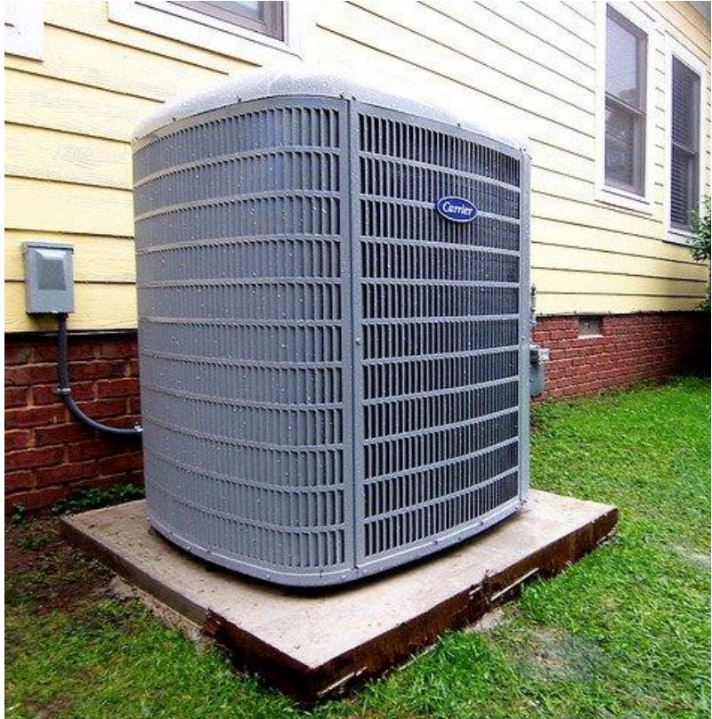
Remote Outside Condenser
